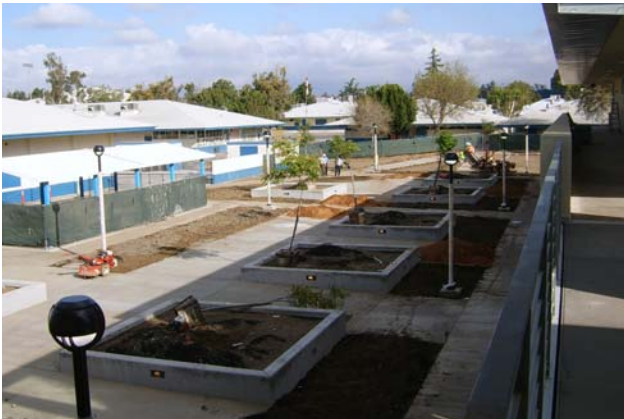
New Interior Courtyard (landscaping is being completed as we go to print!)
