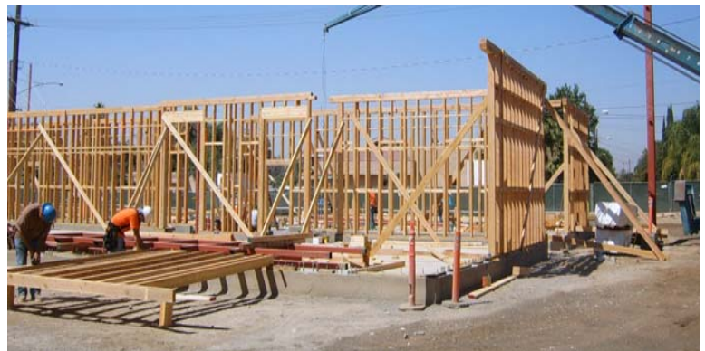
September 2011—With concrete foundation slab poured and cured, rough framing of first floor science building is underway
