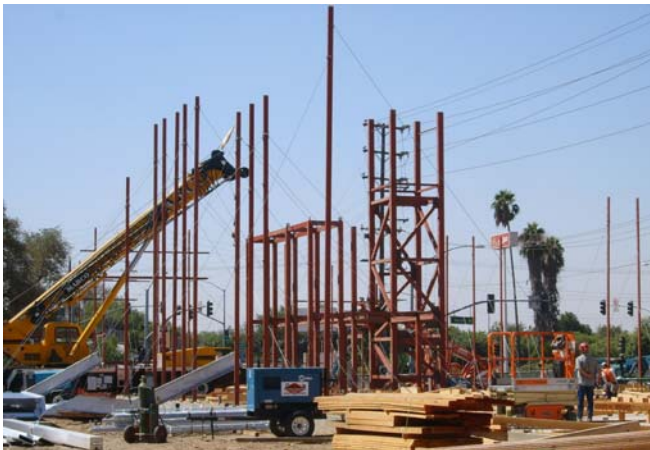
August 2011—project goes vertical with placement of structural steel for stair/elevator tower
