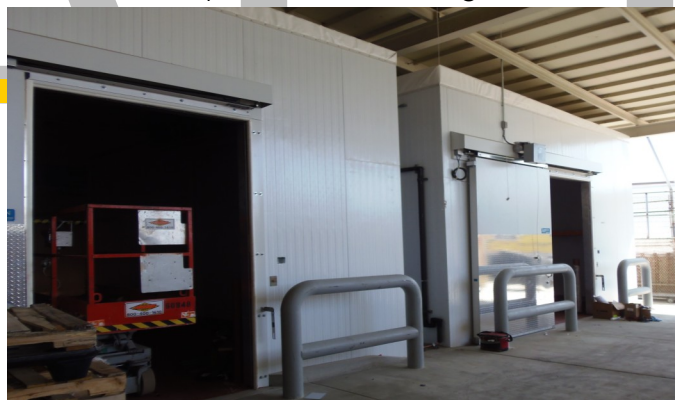
Warehouse Walk-In Freezer
