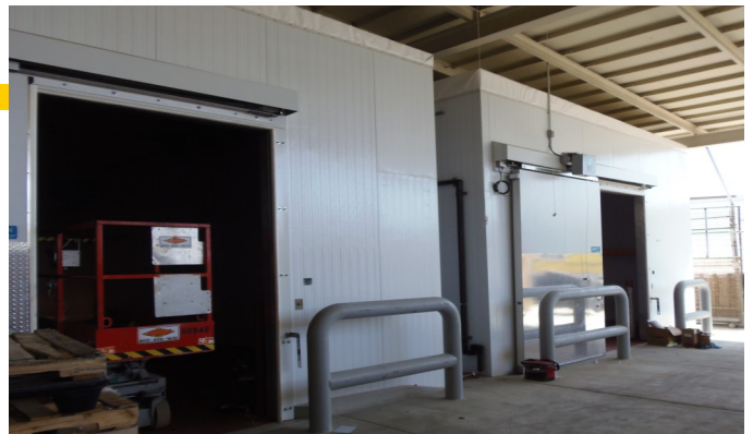
Warehouse Walk-In Freezer
