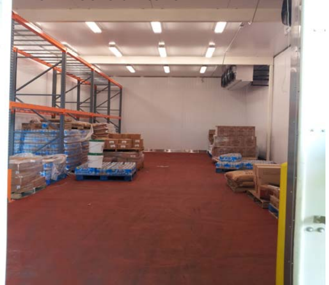
New Freezers Interior
