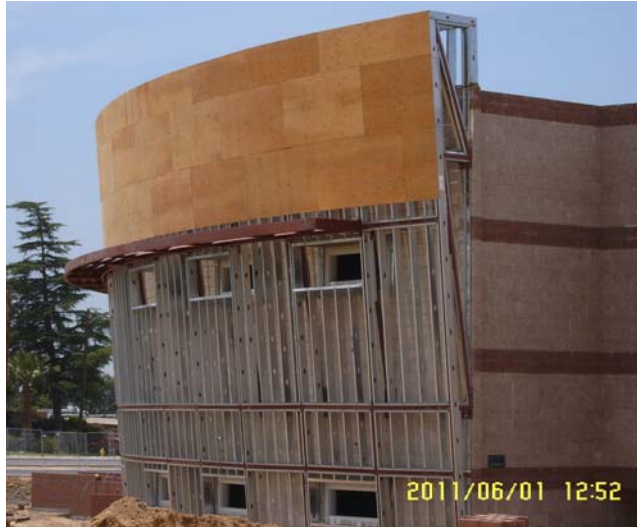
GRAND TERRACE HIGH SCHOOL TOTAL BUDGET: $121 MILLION (Increment 1—Base Campus) CONSTRUCTION: 61% COMPLETE (+1%)
